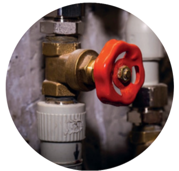
mains water connection
